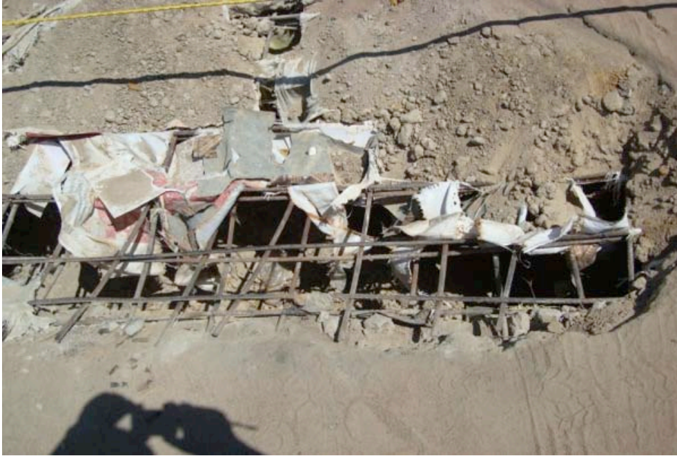
Poorly constructed box culvert
