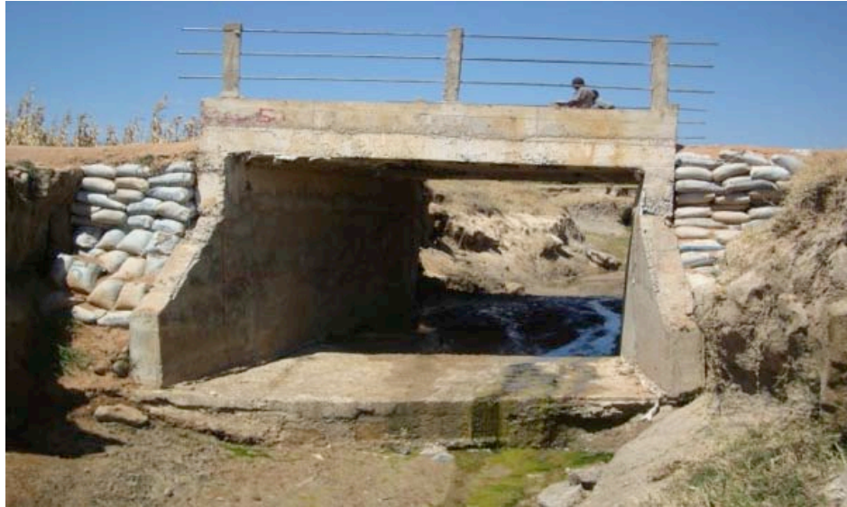
Poorly designed and constructed bridge
