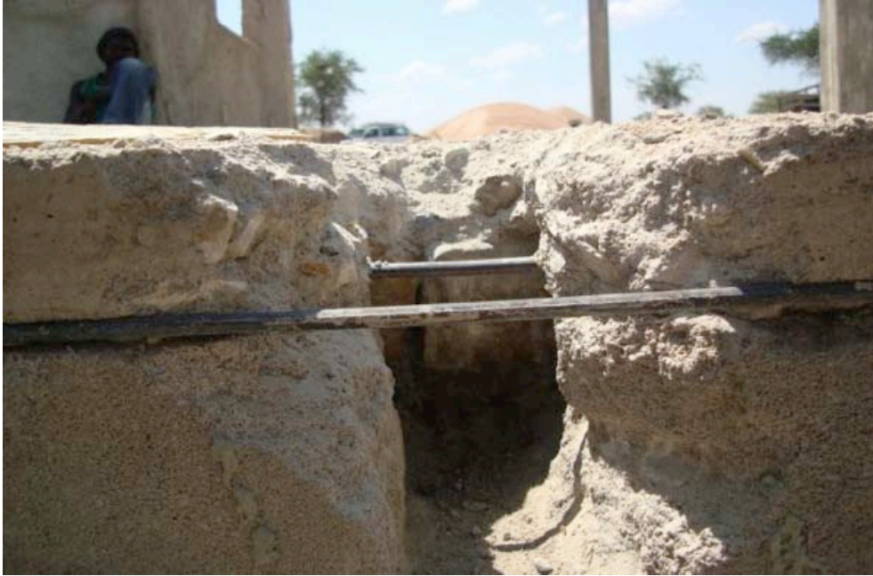
Poorly constructed ring beam
