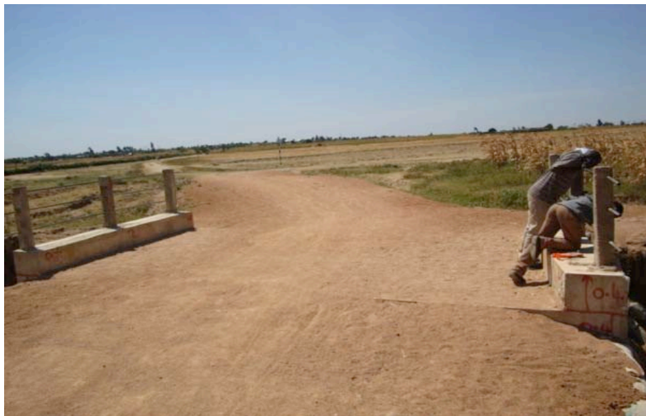
Poor road alignment setting
