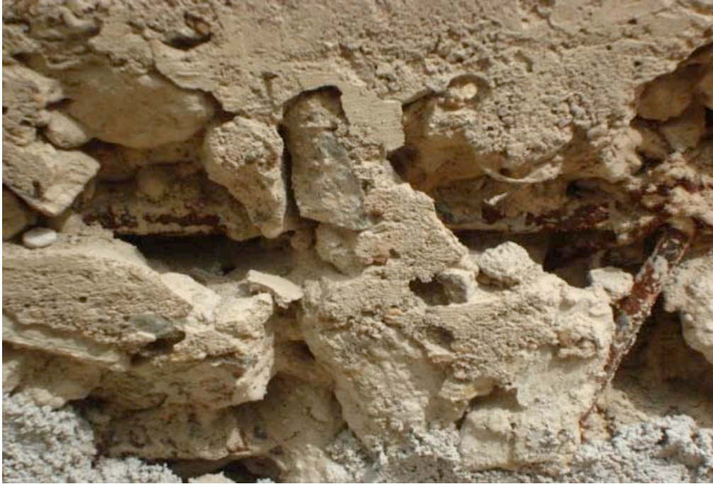
Poor workmanship on a constructed box culvert
