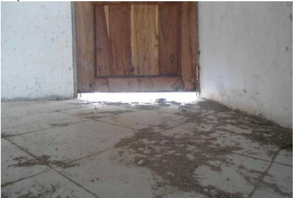
Poorly constructed door
