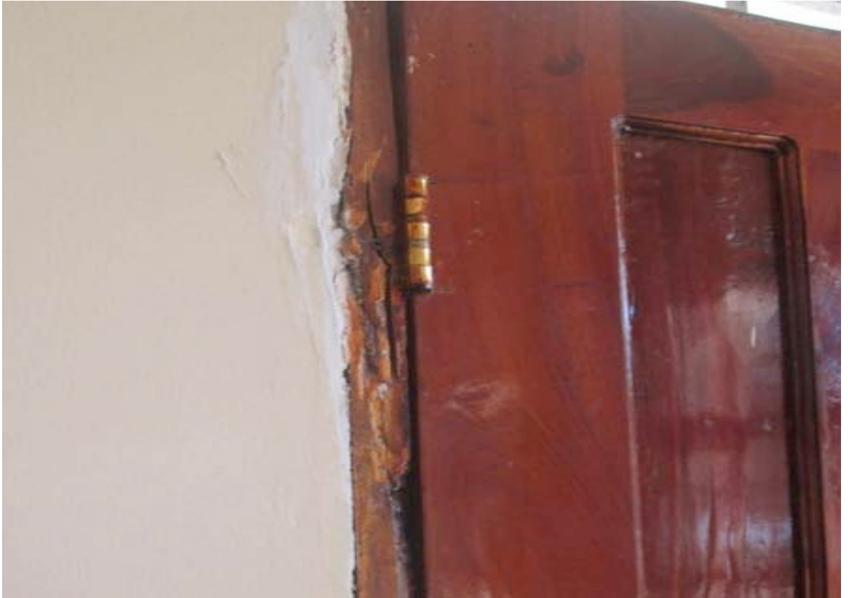
Poorly constructed door
