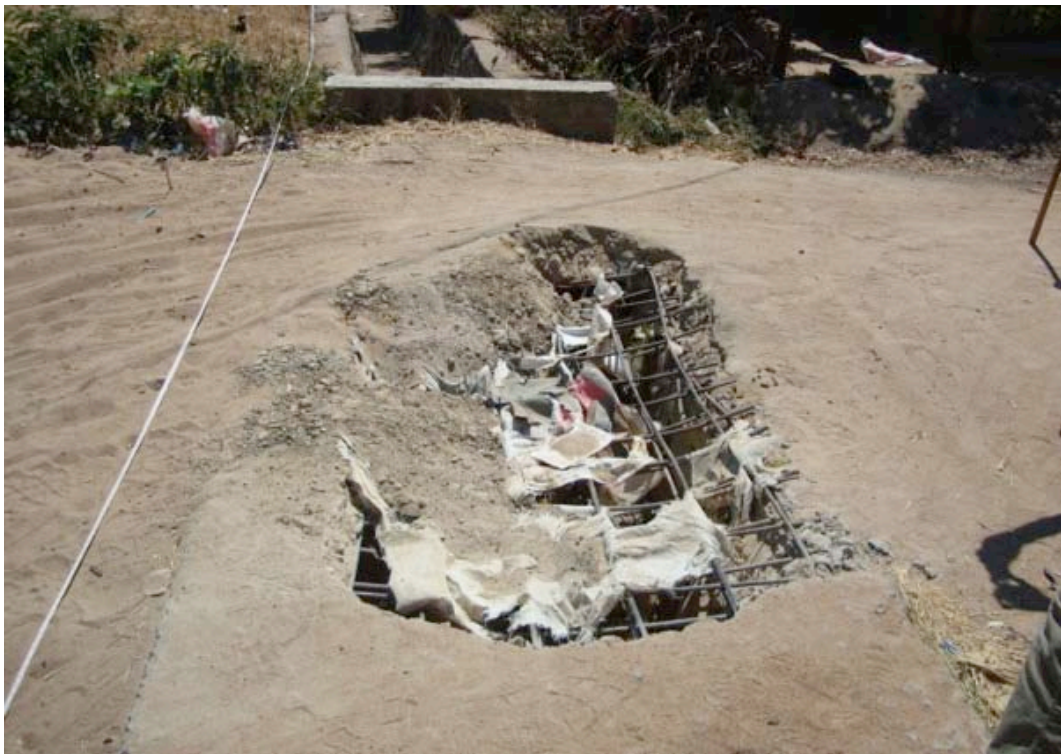
Poorly constructed box culvert
