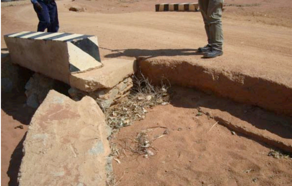
Inadequately designed box culvert
