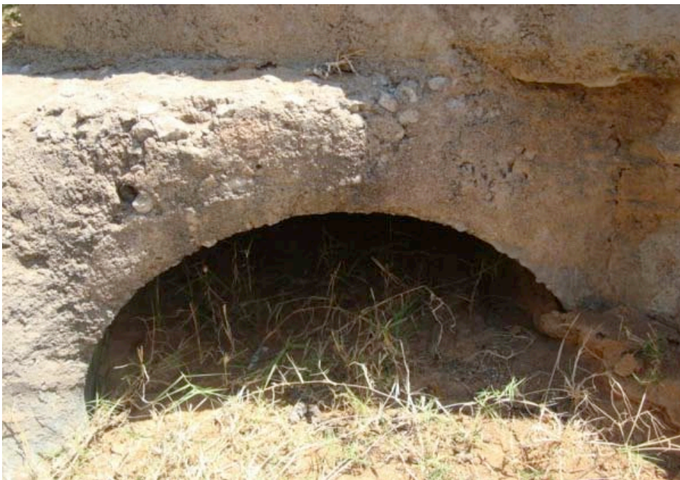
Poor invert level setting
