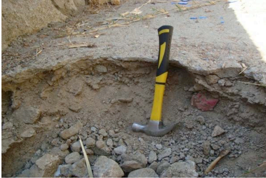
Poorly constructed open drain
